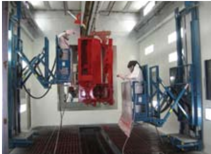
Paint Booth: 3-Axis Lift System for Agricultural Equipment Manufacturer
